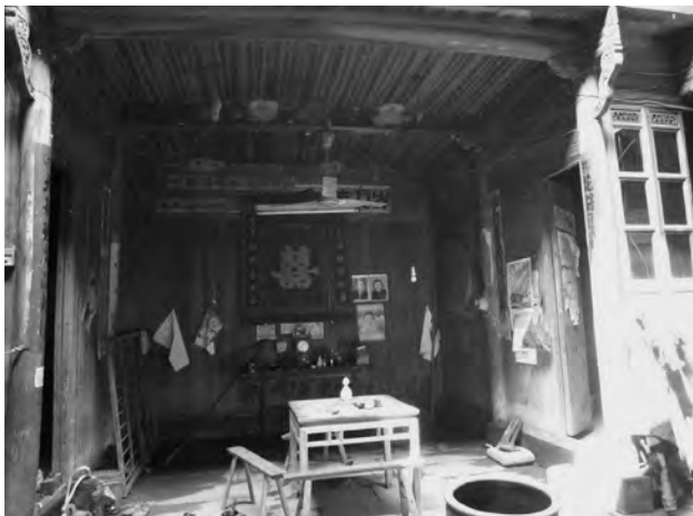
FIGURE 8. The main hall of this house, similar to the hall in Yin Yu Tang, retains traces of both family and social history from the 1970s. However, the deteriorating structure has made the living condition less than desirable. Photo by author.
