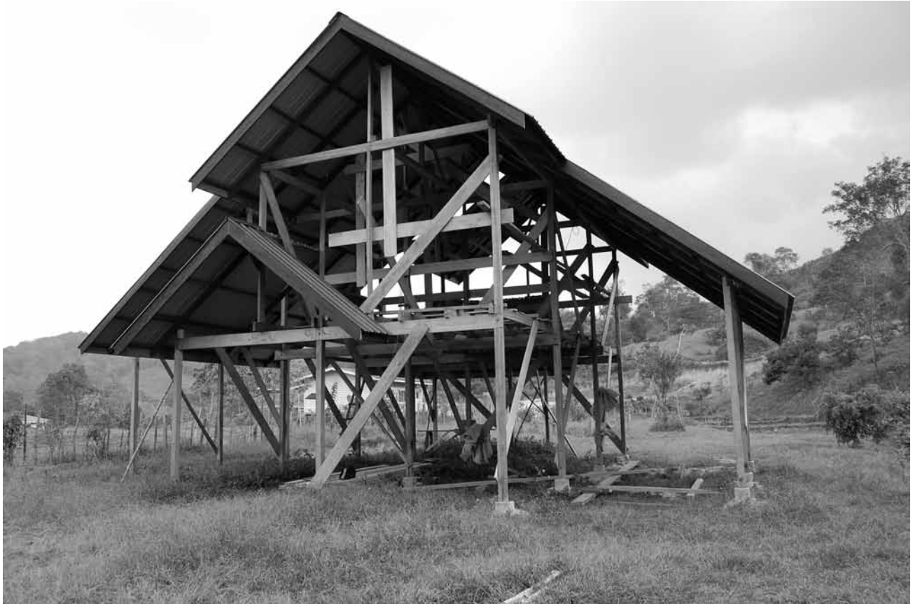
FIGURE 14. Ganang's innovative new house under construction, 2009. The roof shape is inspired by tourist images of Alpine lodges. Photo by author.
