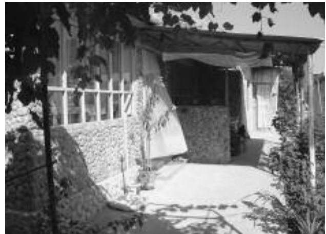
FIGURE 7. Example of house where the original veranda has been closed, while a bower has been improvised in front of the house. Vasile Egor's house, 2 Mai, 2006.
