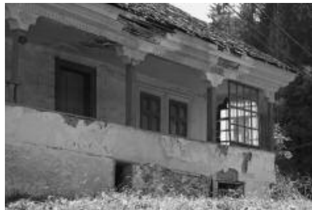
FIGURE 5. Abandoned house in Dambovicioara, Prahova, 2007.
