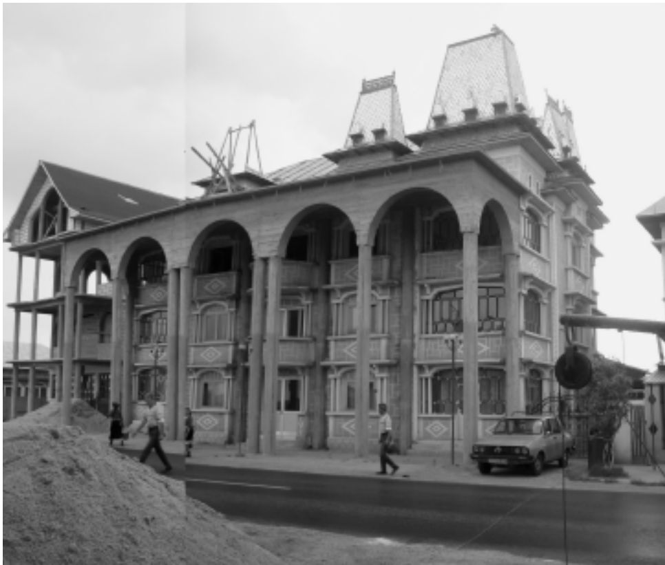
FIGURE 12. Residence under construction in Buzescu. The colonnade is applied on top of the old facade, blocking existing windows, leaving decorative dormers still visible in the back.
