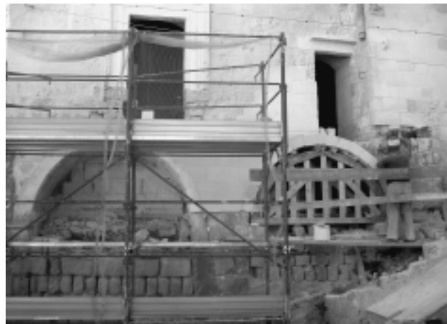
FIGURE 15. Using the traditional method of wooden centering, a mason rebuilds a collapsed barrel vault in the Sassi. Photograph by author, 2003.
