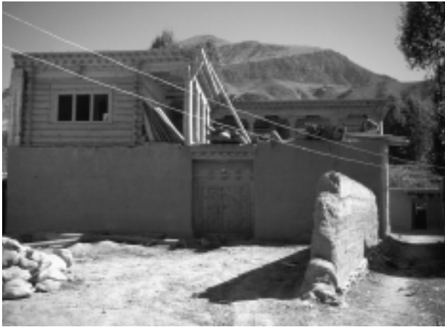
FIGURE 8. Old methods and forms are maintained in this lov benka house under construction. Such buildings using traditional construction materials and methods are becoming increasingly costly, however, due to a lack of local timber since the institution of a logging ban by Chinese authorities. (Photo by author, 1999.)
