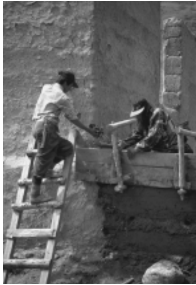
FIGURE 11. Traditional rammed-earth construction is still undertaken for repair and maintenance in Bengda. (Photo by author, 1999.)
