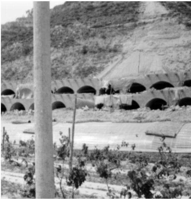
FIGURE 5. New yaodongs under construction. This view emphasizes connectedness with the land. In the foreground is farmland tended by the community.
