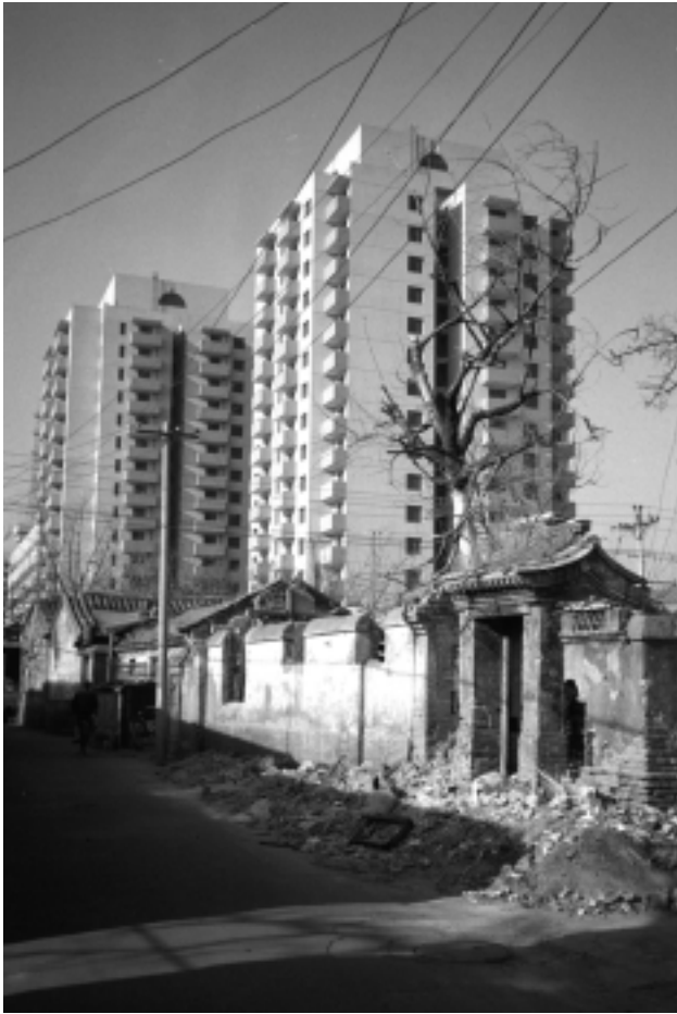
FIGURE 6. Demolition of siheyuan and hutong for new apartment blocks. According to Beijing's master plan, new high-rises are allowed only at the edge of the old city, along the Second Ring Road. But it is not unusual to see eight-story apartments now being built more than one kilometer inside the Ring Road.
