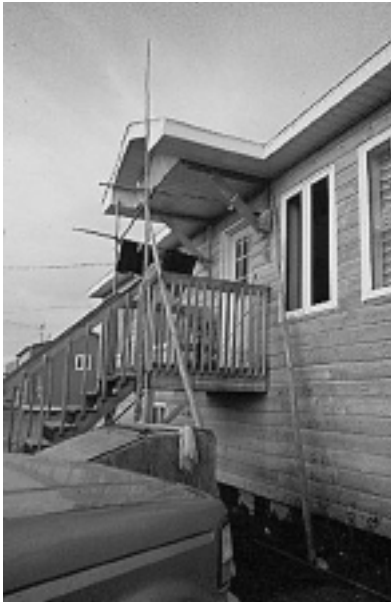
FIGURE II. A roofed porch with a few poles used to hang small game or pieces of meat. Also notice the high level of the ground floor. (Photo by André Casault, 1998.)
