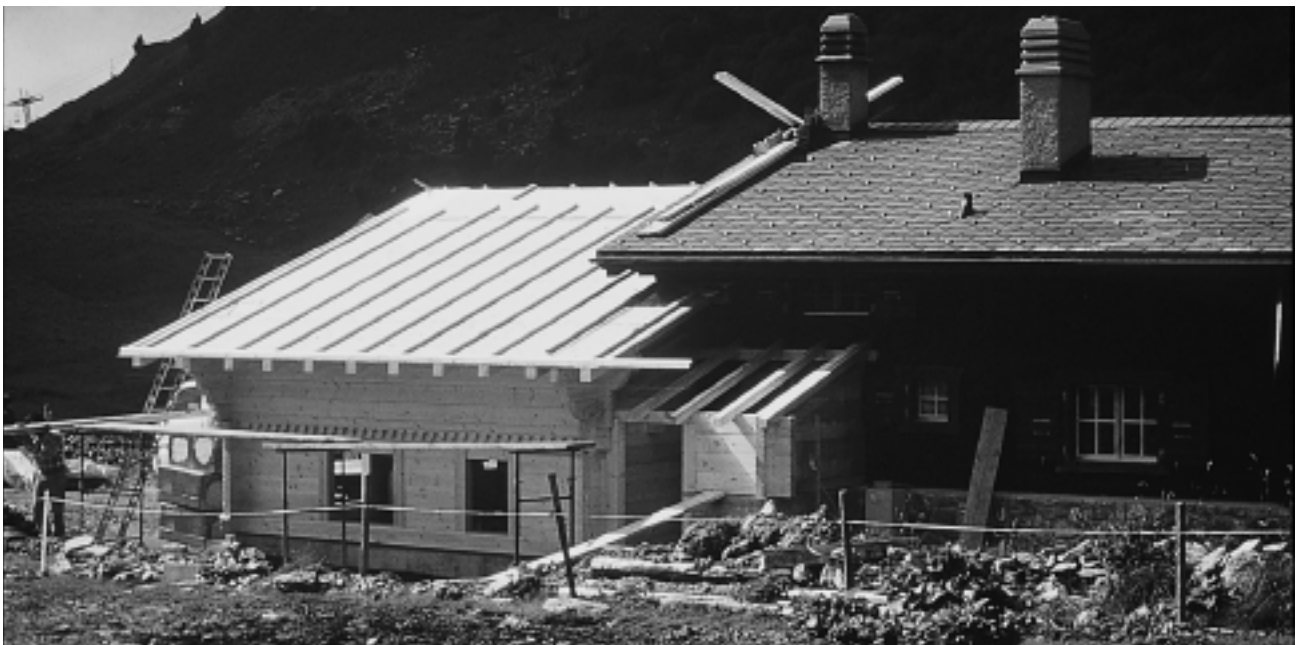
FIGURE 6. Building an extension to a chalet at the Col de Bretaye for rental during the tourist season. Vernacular building techniques are alive and in demand, in this case for the production of luxury chalets at a premium price. Constructor: Daniel Mermod.
