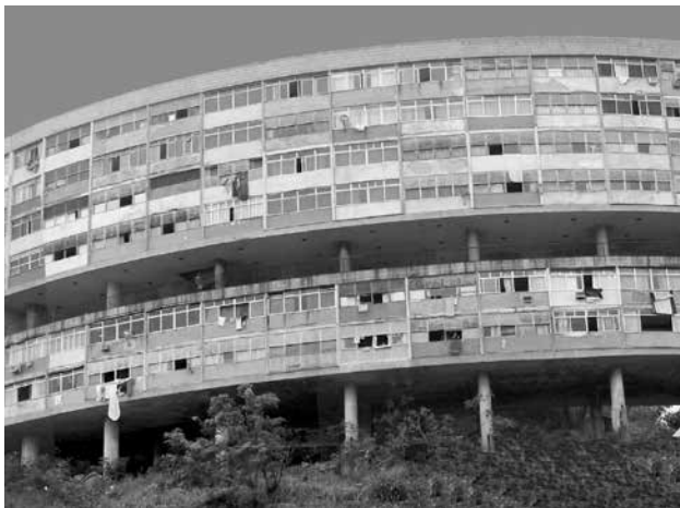
FIGURE 17. Block A before renovation, showing how most of the windows had already been changed by the residents, 2004. Photo by author.
