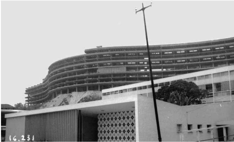
FIGURE 5. In the foreground, the health center and Anísio Medeiros's tile mural. In the background, the concrete structure of Block A under construction, 1951. Source: Arquivo Geral da Cidade do Rio de Janeiro.
