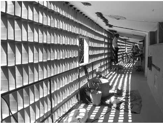
FIGURE 19. Block A apartments corridor, showing a new cobogó panel in the process of being assembled, 2015. Photo by Alfredo Britto.
