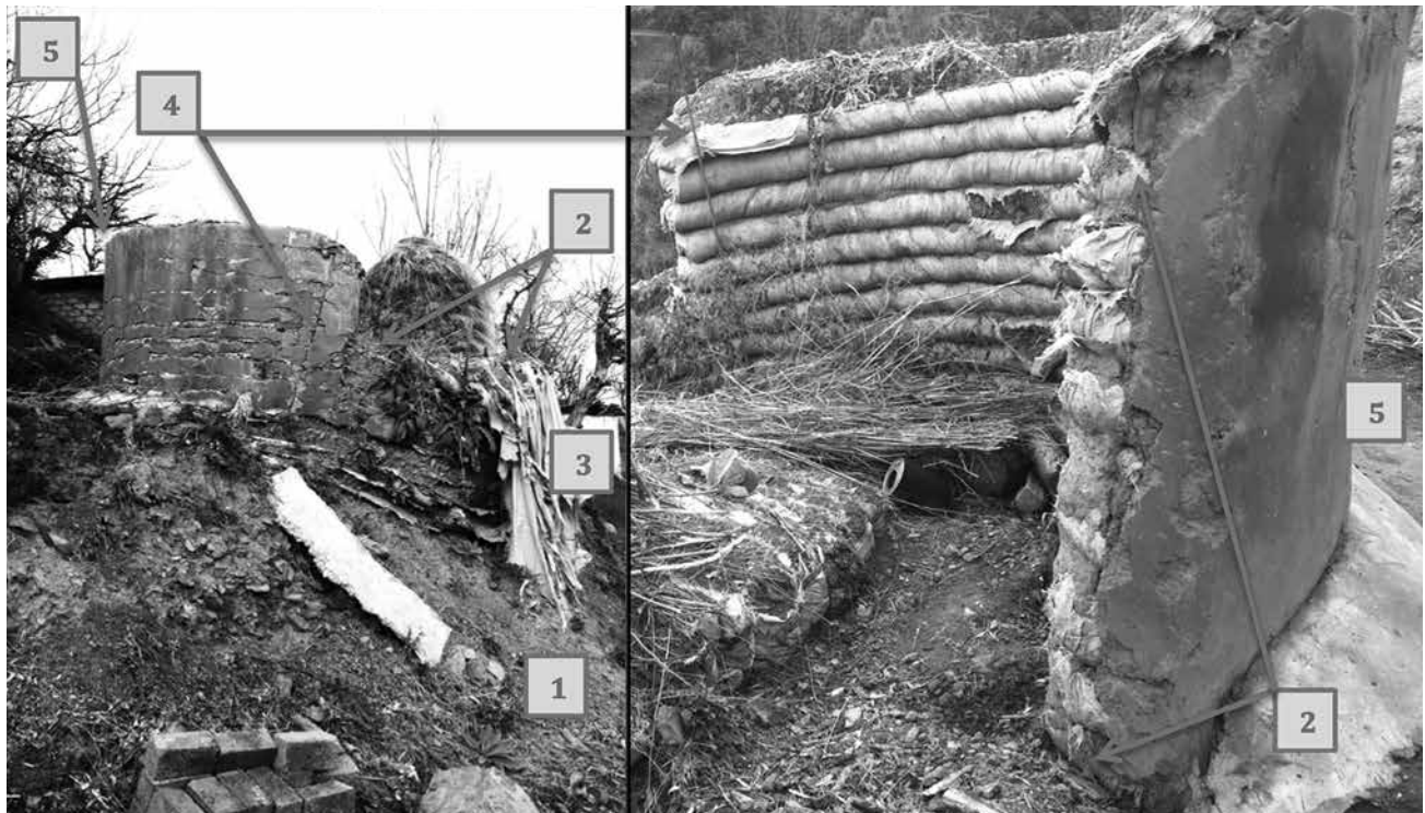
FIGURE 15. Partially collapsed unit found in Dogah-Khairabad. Photos by Mohammad Ashraf Khan.
