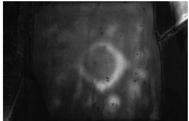
FIGURE 14. Light transmitting slab of marble in the southern wall of the Katholikon.
